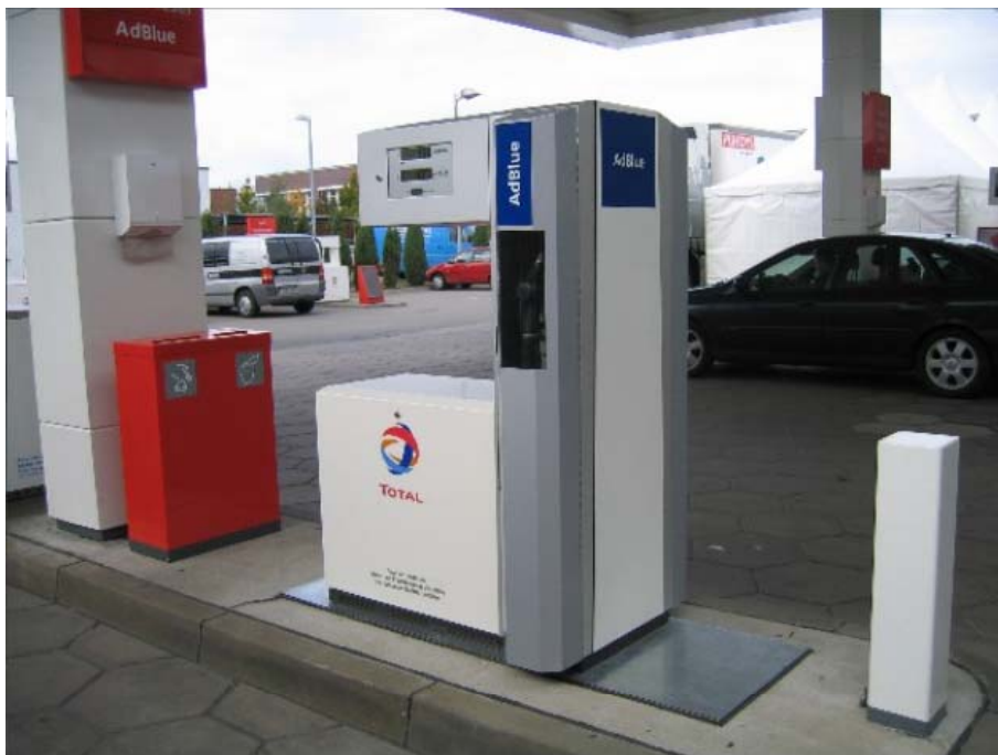
Figure 3: Service Station TOTAL, Berlin Alt-Mahlsdorf
